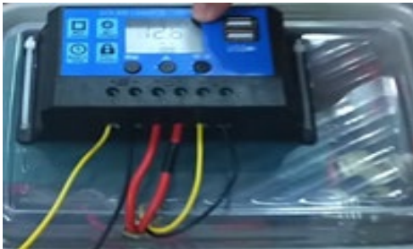
Figure 11: Voltage DC 12.6V to the Inverter
